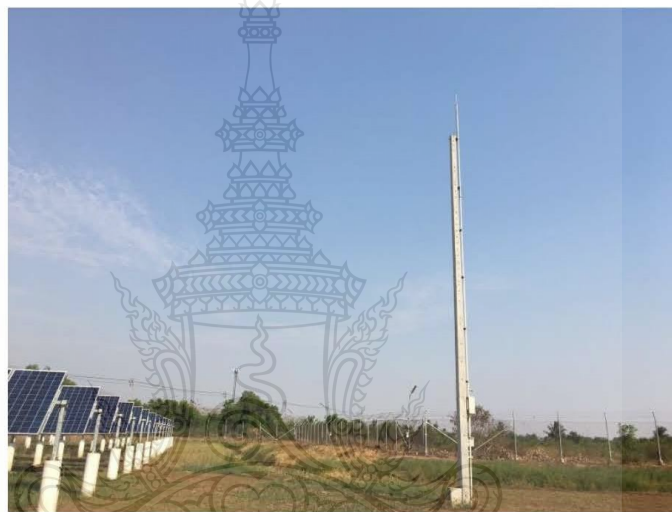
Figure 11. ESE lightning installed at the PV power plant.
