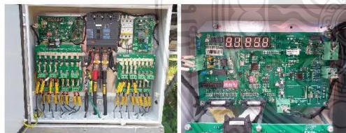
(a) Combiner box (b) Communication data set
