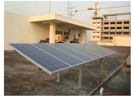
Fig 5 PV Grid Connected System used in this article
