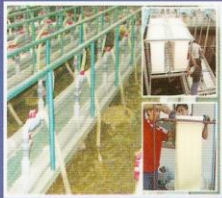
Providing complete wastewater treatment and water recycle system with Membrane Bio-Reactor process
